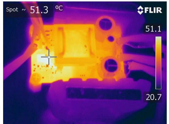
Figure 15. Thermal Image of the ADP1071-1 at 48 V DC Input, Full Load, No Airflow, and 0.5 Hour Soaking Time
