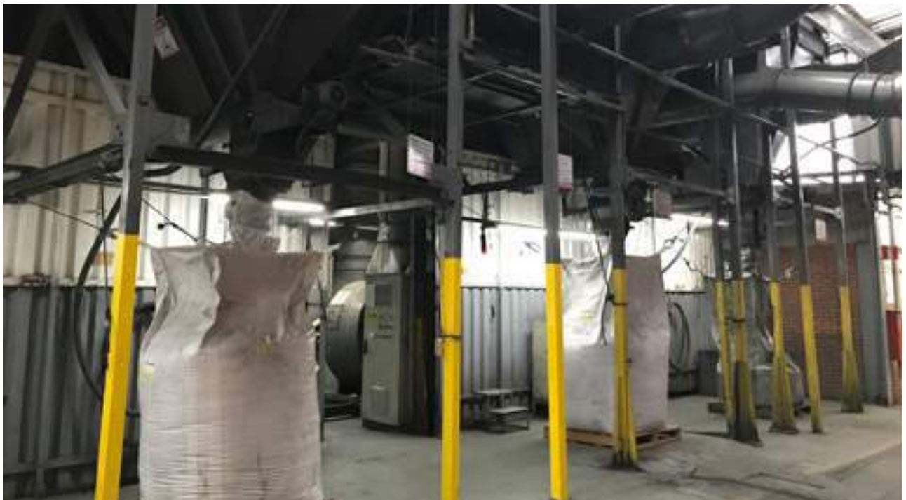
Particulate Material Collection System
