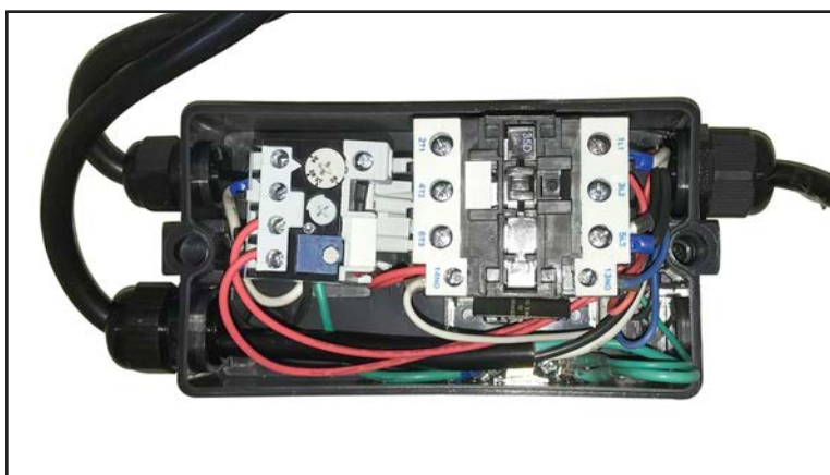
Figure 67. Magnetic Switch (behind control panel).
