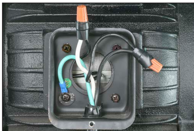
Figure 68. Motor junction box.
