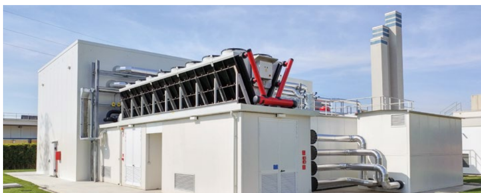
Adiabatic Freecooling Chiller Innovation lab
