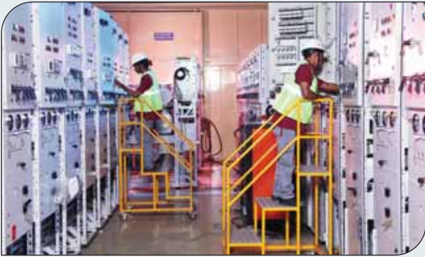
At the Medium Voltage Factory, Goa, localization of global technologies such as compact Switchgear help distribute reliable power efficiently for industrial and urban areas.
