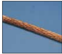
Lightning Protection Cable
