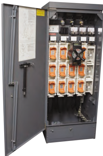
🔧 Outdoor fuse cabinet
