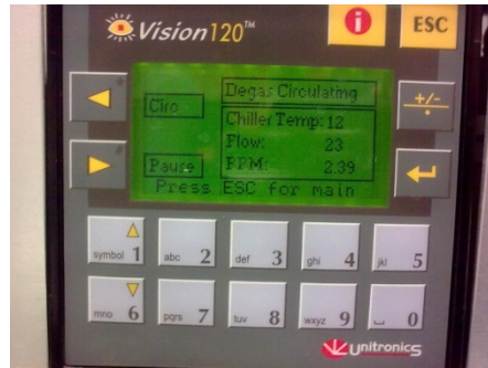
Figure 3-3: Water System Control Panel
