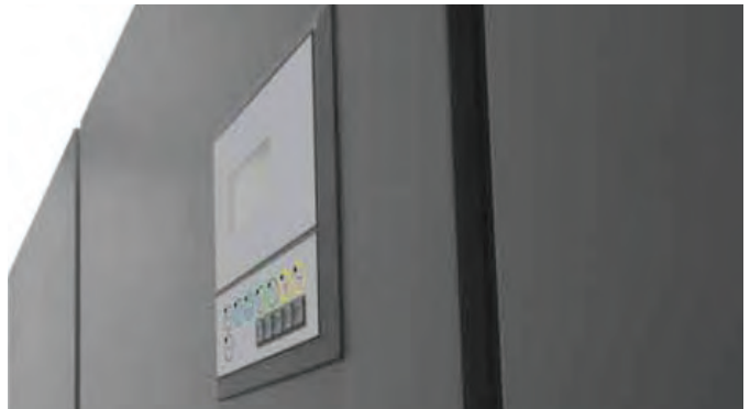
Modulating controller display and keypad
