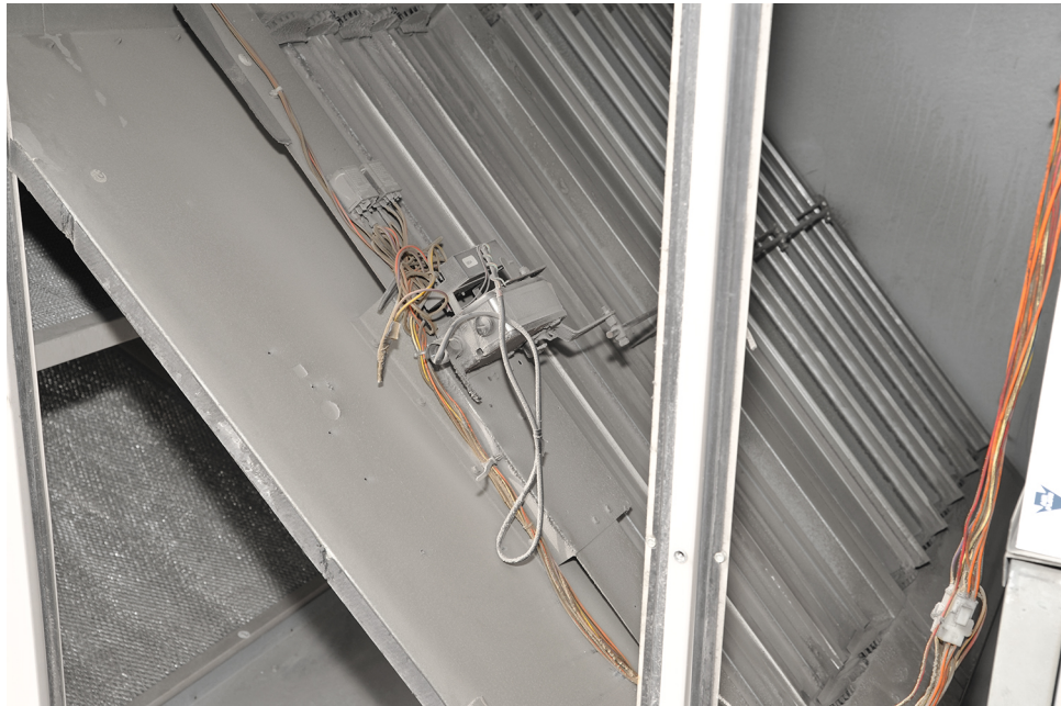
Figure 6. Dusty economizer damper.
