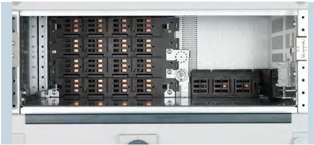
Fig. 4/14: Compartment for normal withdrawable unit in HFD
