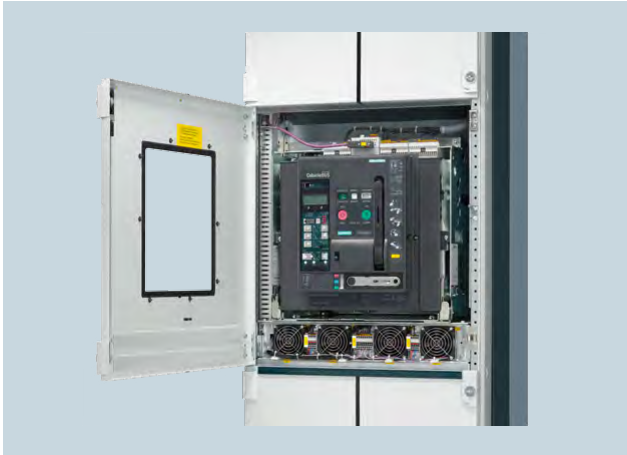
Fig. 3/2: Forced cooling in a circuit-breaker cubicle
