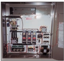
Replacement/Upgrade Starters for Centrifugal Chillers
