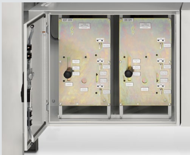
Fig. 19 Central drive cabinets for earthing switches, disconnect and start-up disconnect
