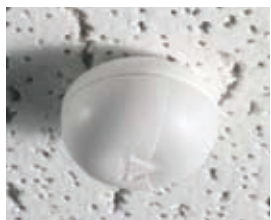
Mounting on ceiling tile
