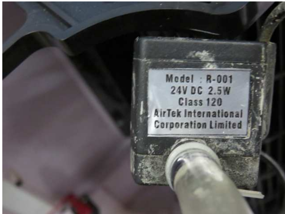
Water pump view
