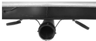
Black/Grey Tank Drain and Valves
