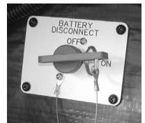
Battery Disconnect Switches
