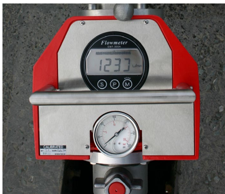
Fig. 4.2 An example of a flow readout and a residual pressure reading. Photograph courtesy of Laois Fire Service.
