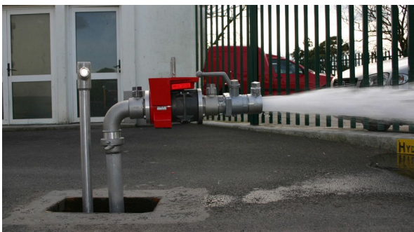
Fig. 4.3 Flow testing with ball valve to facilitate static and residual pressure measurements at Portlaoise Hospital. Photograph courtesy of Portlaoise Hospital Service
