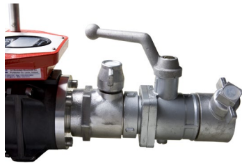
Fig. 7.1 Ball Valve to facilitate static pressure measurements
