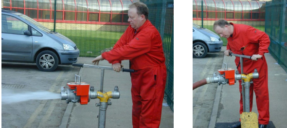
Fig. 4.1 Testing an underground hydrant using a standpipe. Photographs courtesy of Essex County Fire and Rescue Service.
