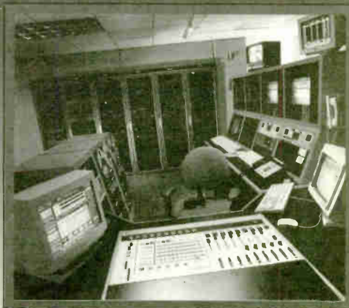
The Master Control Studio, shown right, is one of seven Arrakis studios in Sony's Manhattan network origination center for SW Networks.
