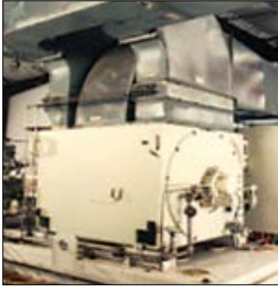
This 3500HP, 3/60/4000 Volt, 3600 RPM, TEFV horizontal motor is powering a pump on an oil pipeline.
