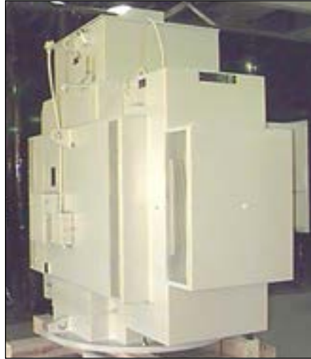
HP: 600 RPM: 360 Frame: V9240 Enclosure: WPII Application: Centrifugal Pump Industry: Coal Fired Generating Station
