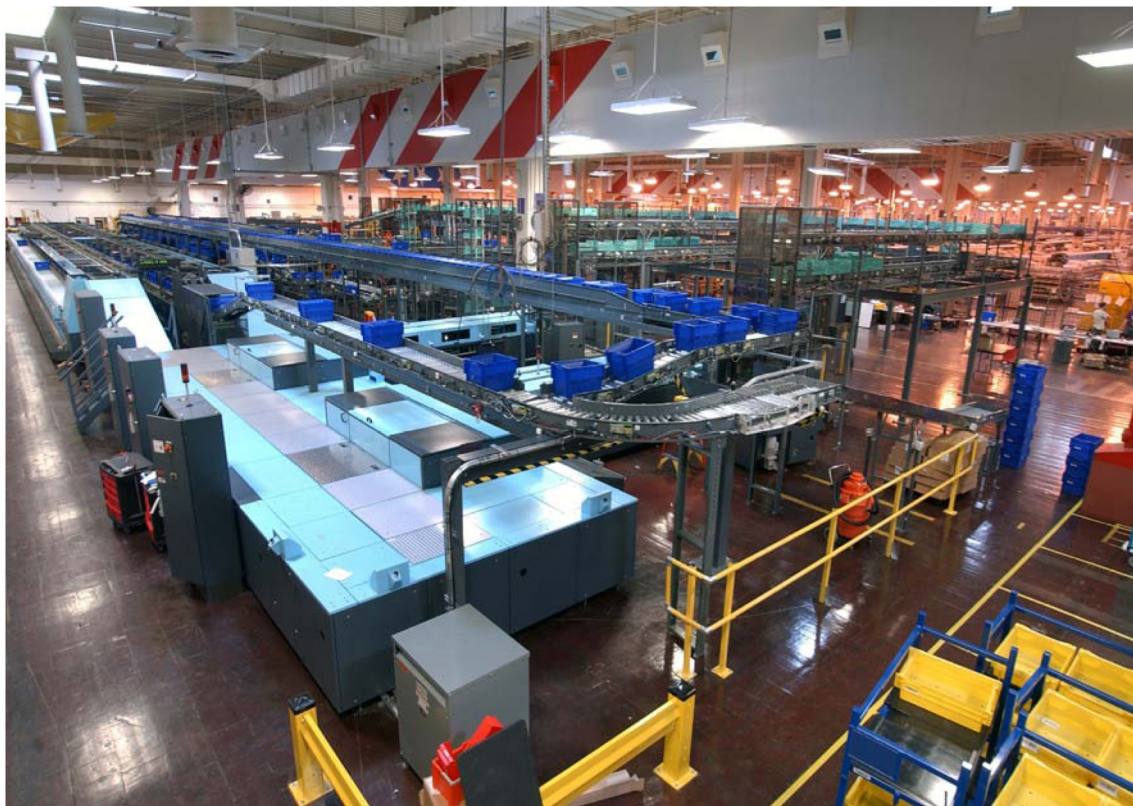
Figure 14: Flats Sequencing System
