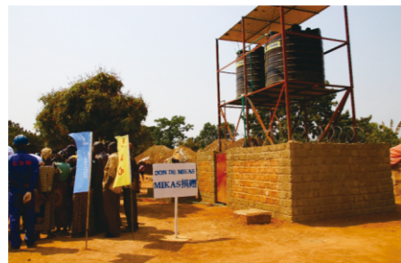
MIKAS-funded Solar Water Well in Village
