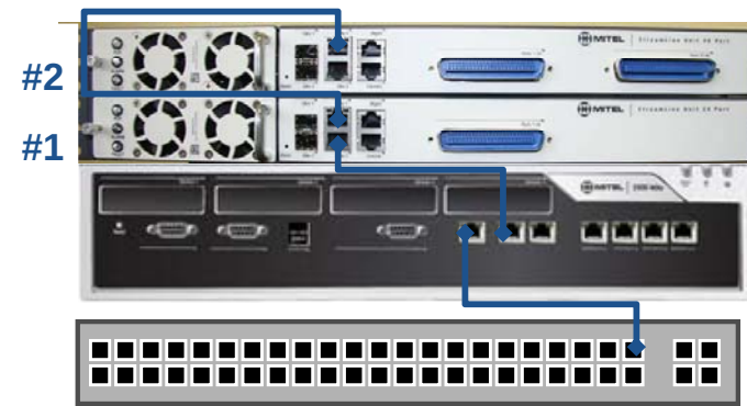
Consolidating data switch, router, firewall
