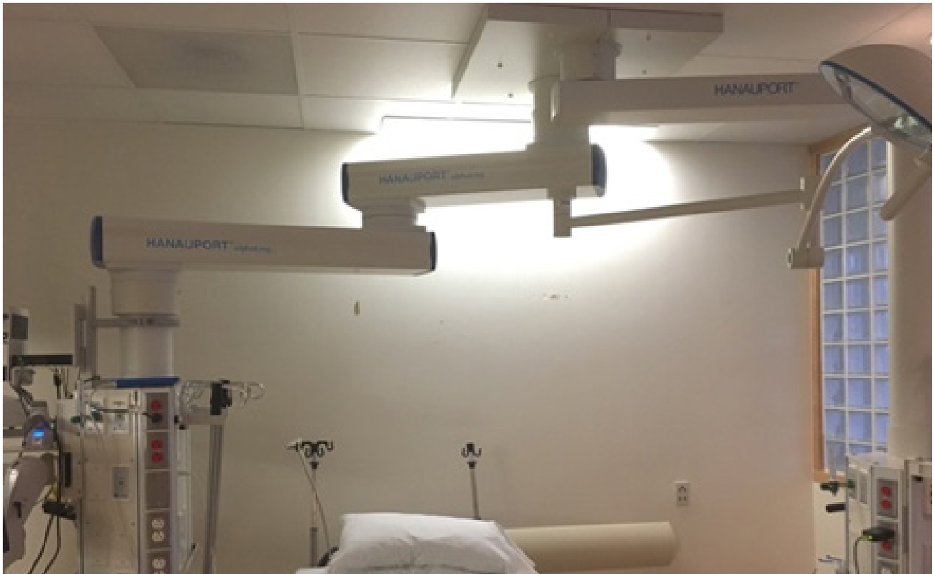
Figure 3 – Emory University Hospital Neuro ICU. The overhead boom in these rooms facilitates easy access to the head of the bed, which is imperative for a Neuro ICU. Patient lifts were not incorporated into most of these rooms
