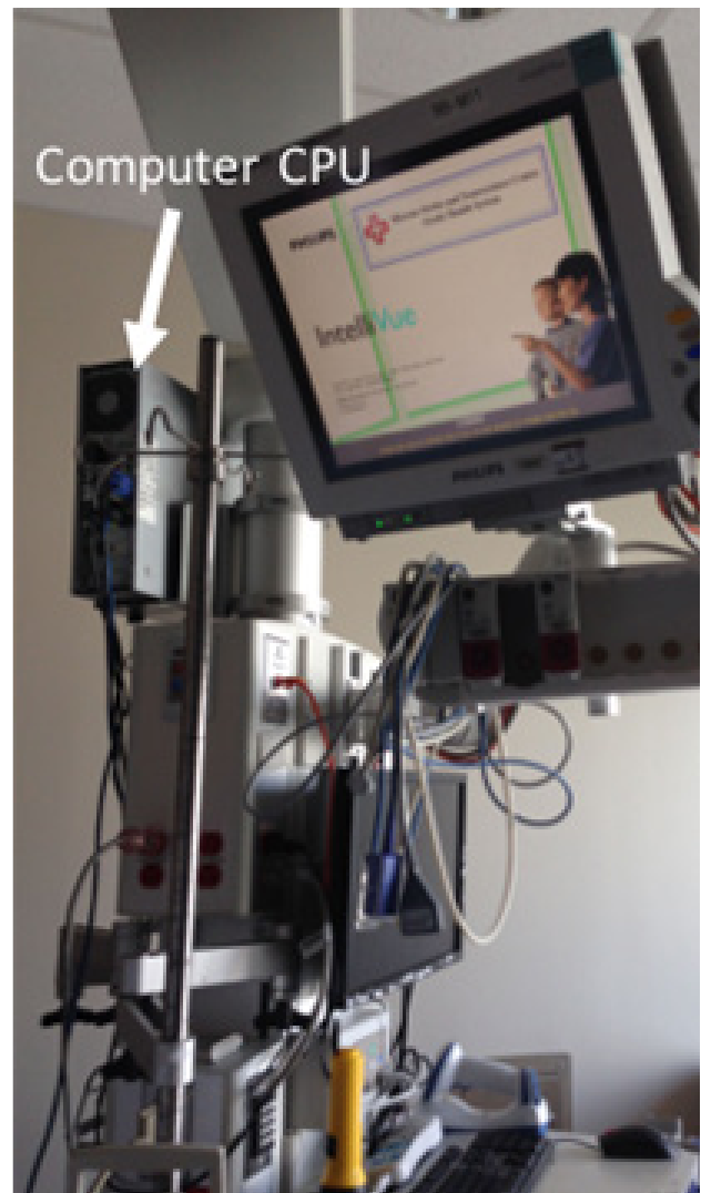
Figure 1 – Boom at the Marcus Stroke and Neuroscience Center. The CPU is mounted high on the column and not well secured.
