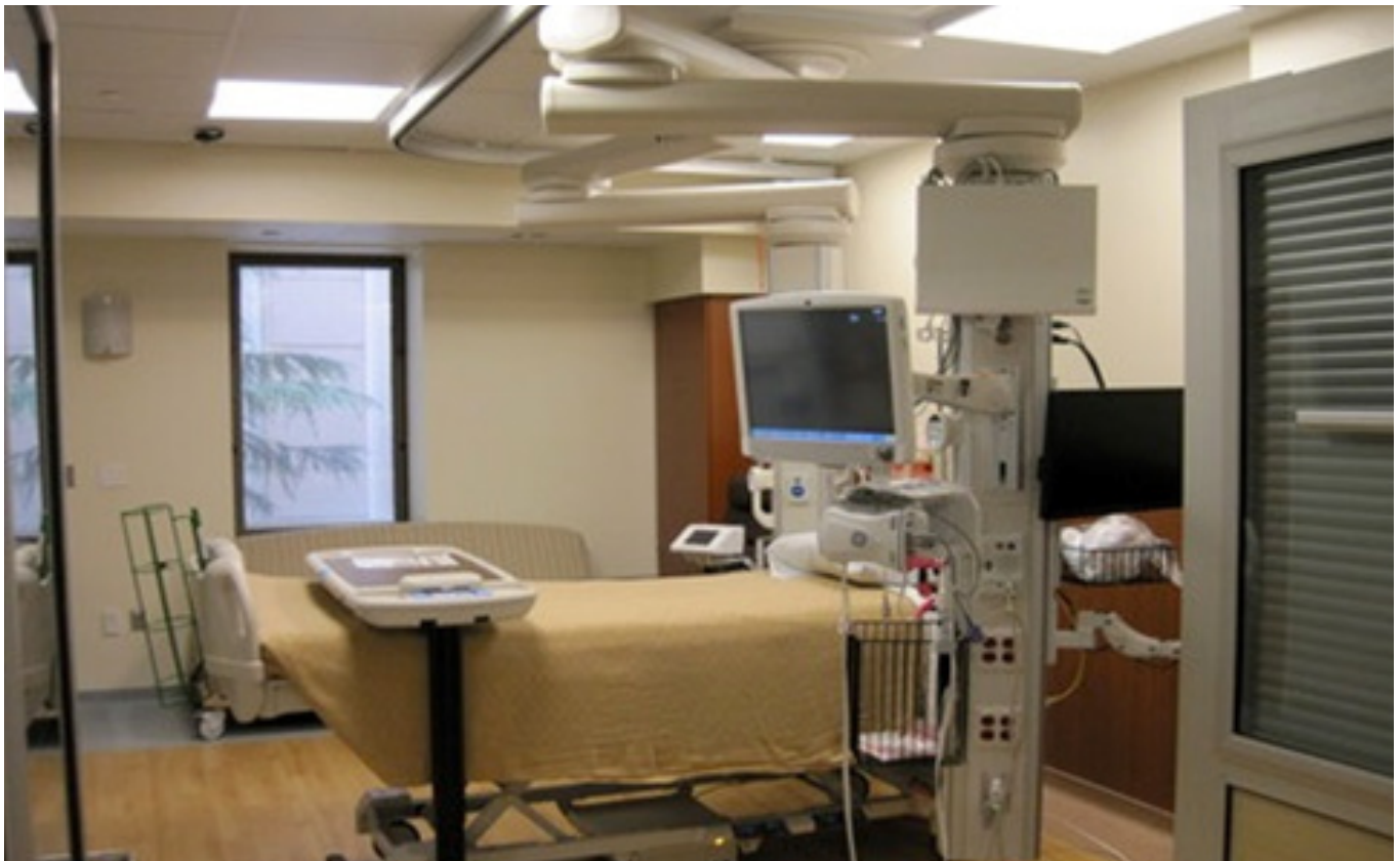
Figure 2 A and 2 B – Emory University Hospital Midtown Surgical ICU. Top figure shows the ceiling track for the patient lift which is over the bottom third of the bed. The bottom image shows how the articulated arms of the boom overlap the patient lift track and therefore need to be pushed out of the way in order to use the patient lift.
