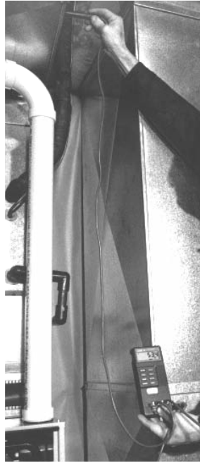
FIGURE 48 TEMPERATURE RISE MEASUREMENT
