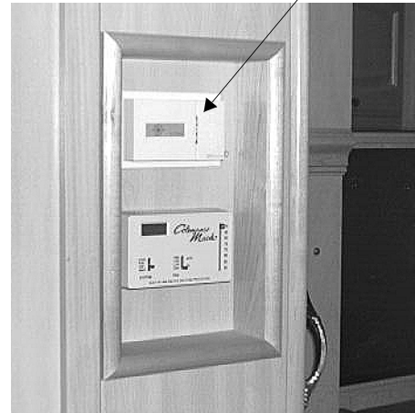
Power Ventilator Thermostat - Galley
