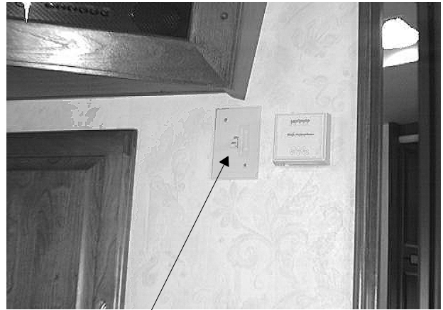
Engine Block Heater Switch
