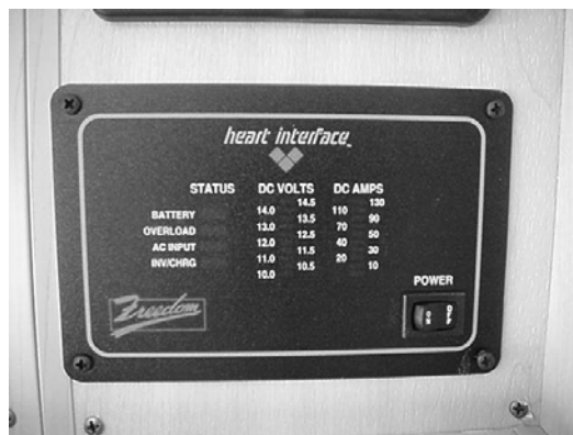
Inverter/Charger Remote Panel
