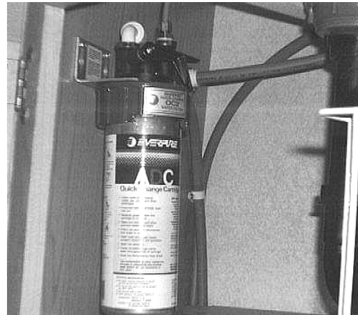
Water Filter Assembly - Below Galley Sink
