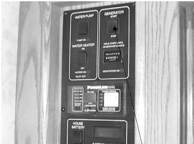
Generator Switch and Hourmeter
