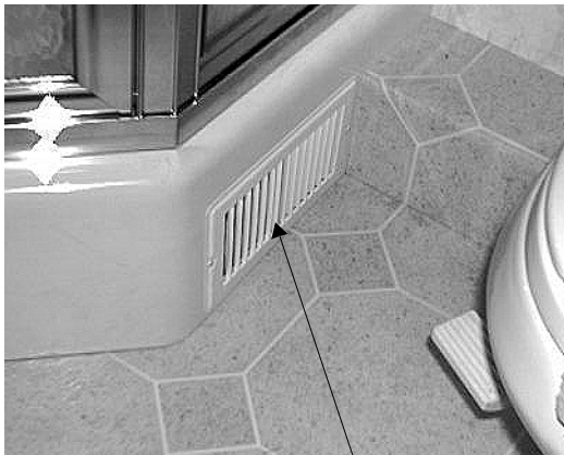
Shower Line Drain Access (behind air return grate in shower base)
