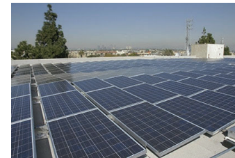
Solar panels on the roof of SPE's headquarters
