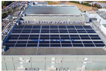
Solar panels installed on the roof at Kumamoto TEC
