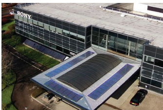
Solar panels on the roof and ground of the UK TEC TEC
