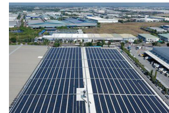
Solar panels on the roof of STT-C
