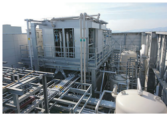
Wastewater recovery facilities for water used for combustion treatment to remove exhaust gas
