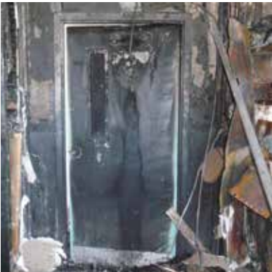
These photos illustrate the value of a code-compliant fire door. This door prevented the spread of fire from a maintenance area to the rest of the Robert Moses Nature Center. It's easy to imagine what the outcome would have been if the door had been propped open.
