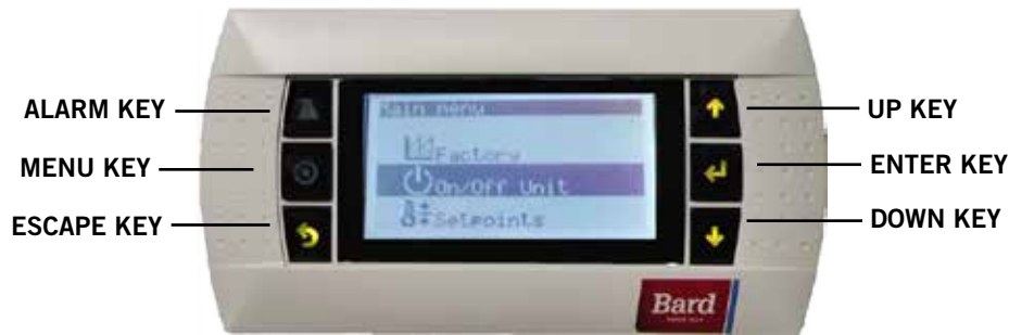
FIGURE 1.27 Bard-Link™ Controller Display
