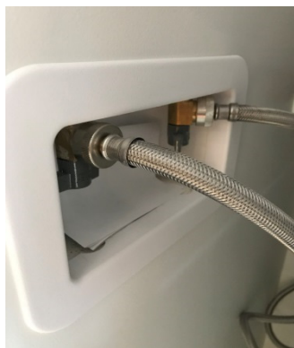
Water Shut-Off Valve
