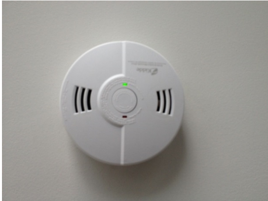
Smoke and Carbon Monoxide
