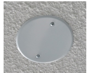
Ceiling Electrical Box
