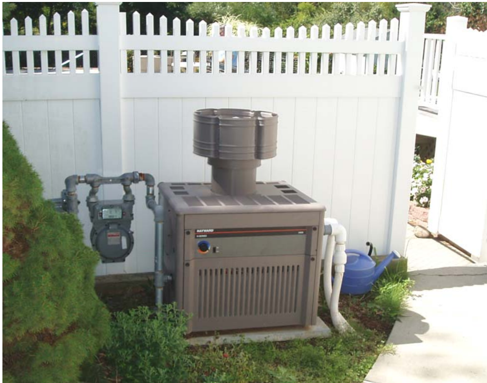
Figure 2 Hayward H-400 pool heater at the Southold, NY field test site
