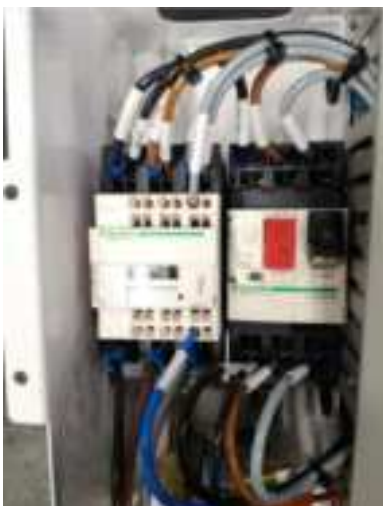
Figure 18: Main switch & overload protection AGL_Unit_ZXDI_E_Rev02
