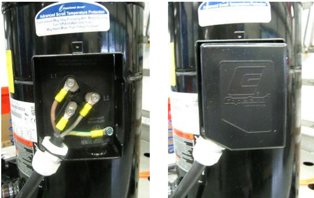
Figure 10: Correct electrical installation with cable glands for IP21 T-box
