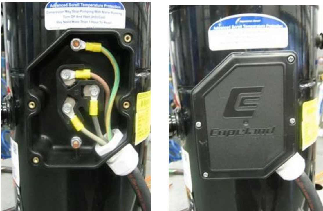
Figure 11: Correct electrical installation with cable glands for IP54 T-box
