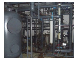
Wastewater reusing system
