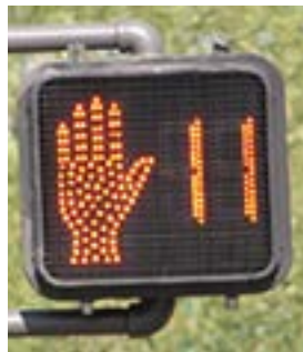
Figure 22. Pedestrian countdown signal. (Source: Resident's Guide for Creating Safer Communities for Walking and Biking ).
