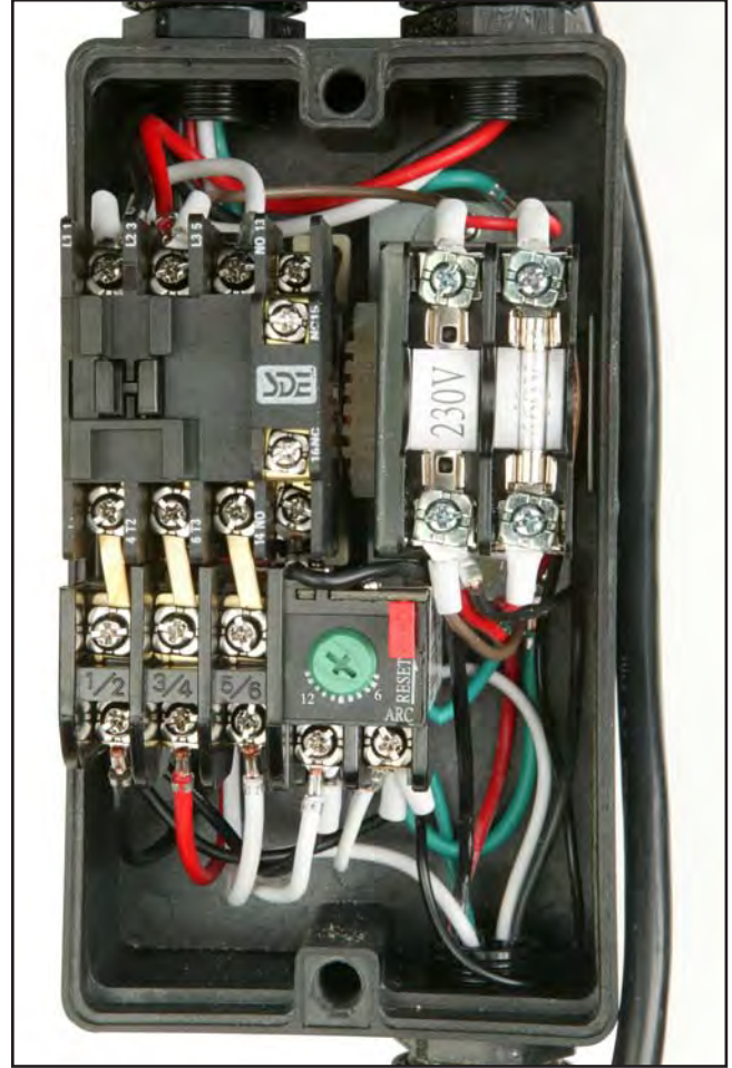
Figure 154. G0652 magnetic switch converted to 440V, 3-phase.
