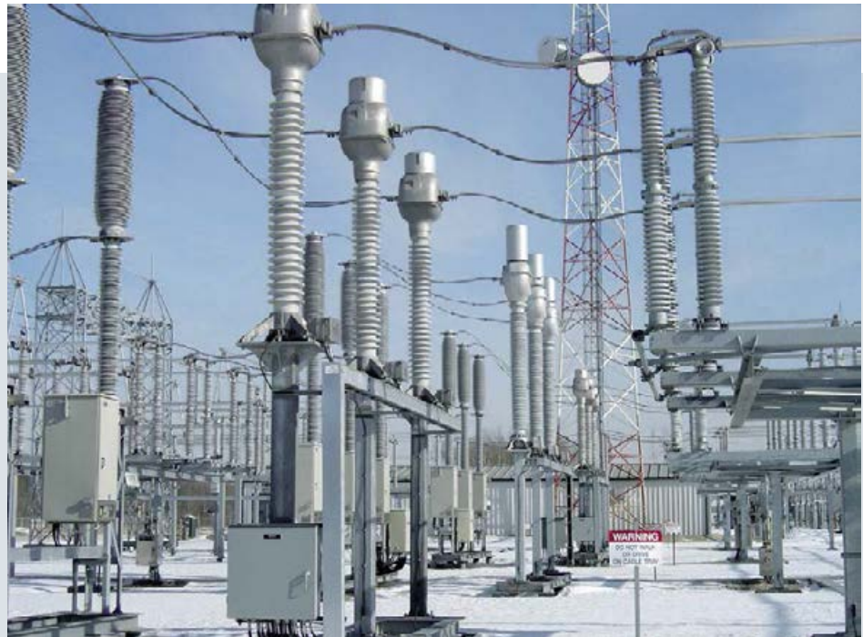
Fig. 47: 300 kV oil-immersed current transformers in Alberta, Canada
