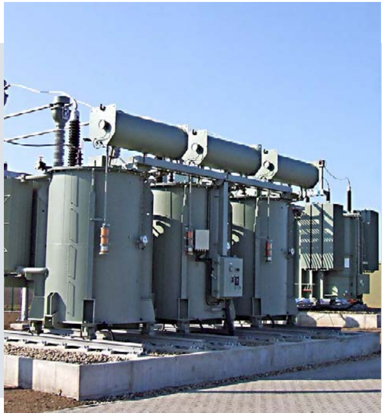
Fig. 70: Variable shunt reactor
