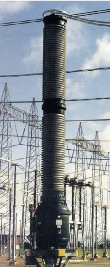
Fig. 46: 765 kV gas-insulated voltage transformer
