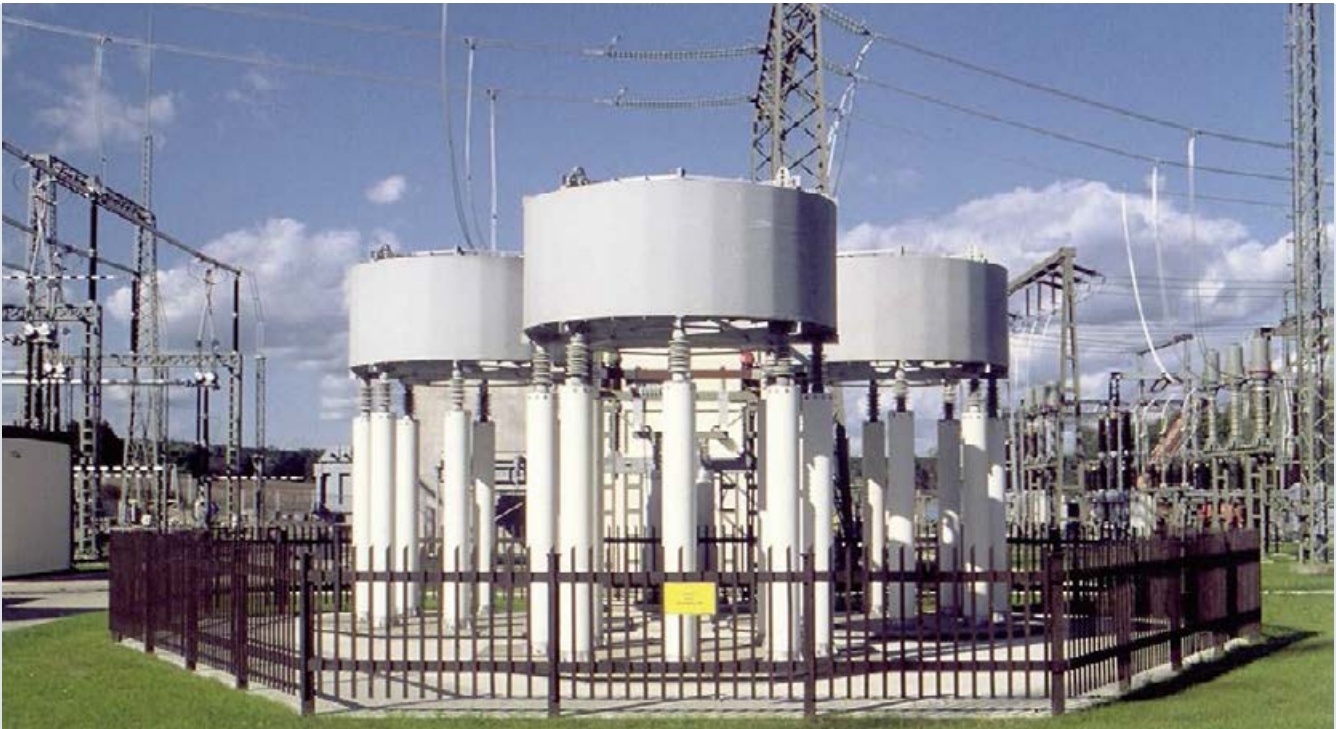
Fig. 67: Tertiary-connected shunt reactors
