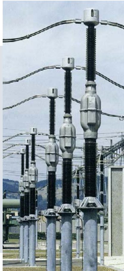
Fig. 49: 420 kV oil-paper-insulated inductive voltage transformers
