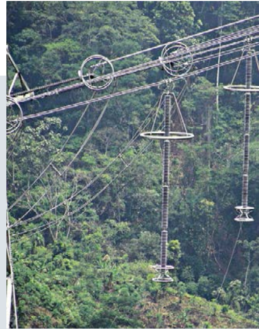
Fig. 35: 550 kV line in Colombia, NGLA solution realized with 3EL2
