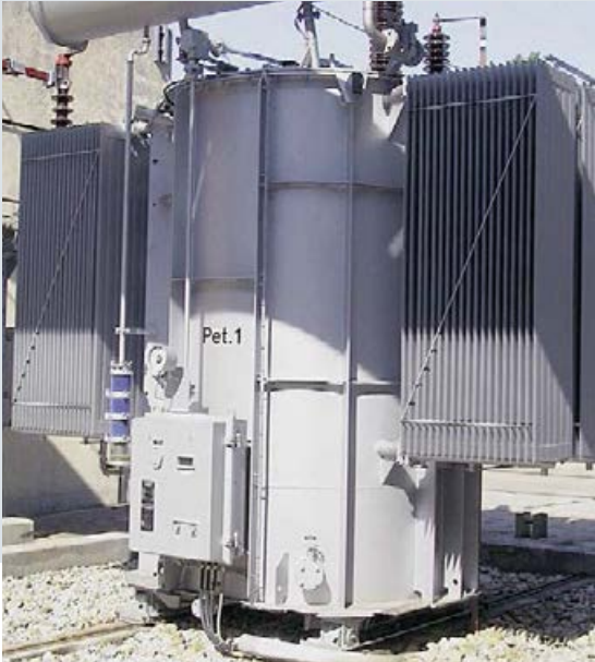
Fig. 69: Arc-suppression coil 110 kV
