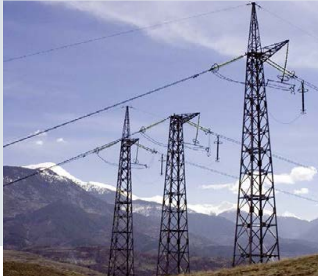
Fig. 34: 400 kV line in Bulgaria, NGLA solution realized with 3EL2
