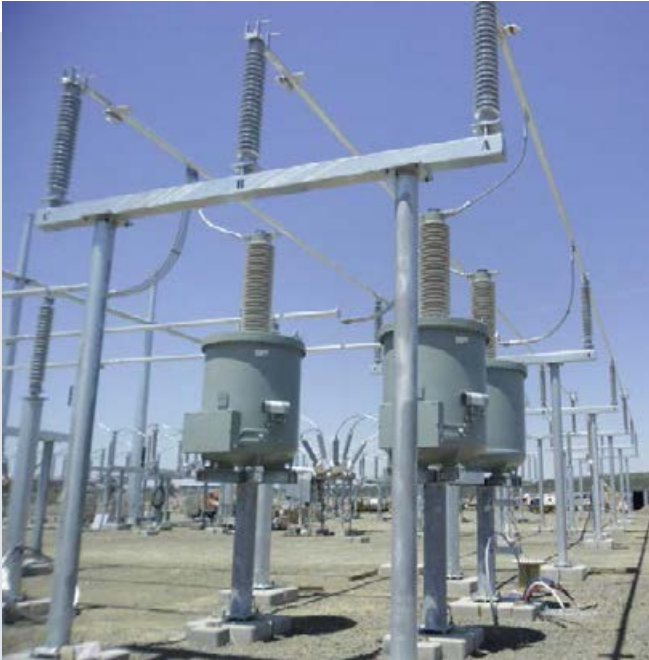
Fig. 61: 145 kV power VT for AIS
