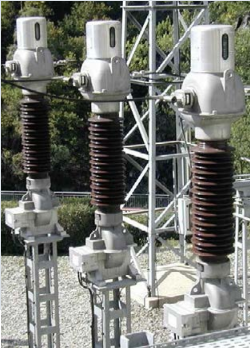
Fig. 50: 550 kV oil-immersed combined instrument transformers
