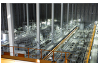
Expanded Multi-Radionuclide Removal System (MRRS)
