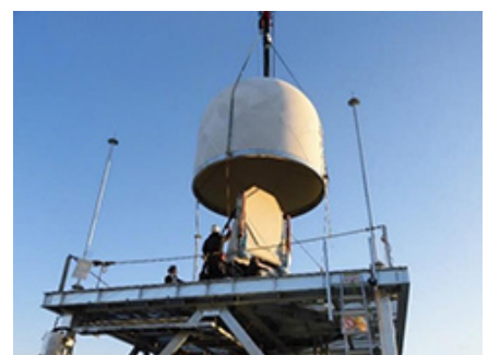
MP-PAWR at time of installation at Saitama University (before covering the antenna with a radome)
