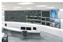
Supervisory Control And Data Acquisition Systems (SCADA)
