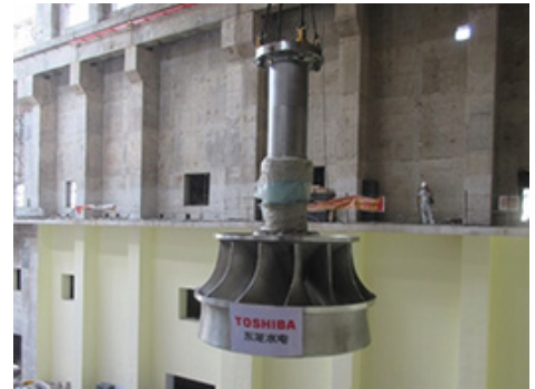
The hydro turbine installed at Trung Son Hydro Power Station
