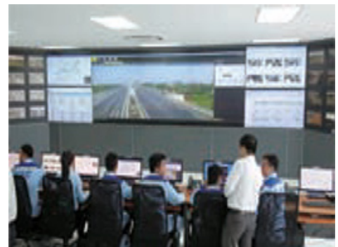
An expressway traffic control center in Vietnam that has started operation of Intelligent Transport Systems
