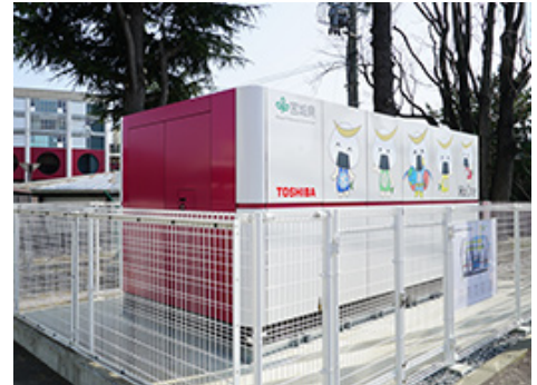
H2One™, Hydrogen energy supply system for Rakuten Seimei Park Miyagi
