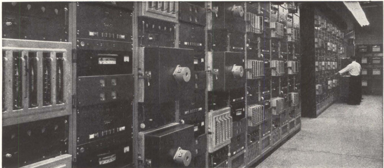
Banks of racks are used for d-c dissipation tests of transistors. Small detachable ovens with individual temperature control can be placed over selected racks for testing at elevated temperatures. Special techniques are used to prevent the testing operation from introducing failure from wrong connections, overloads or voltage transients
