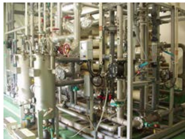
Reverse osmosis (RO) membrane device (Toyooka Factory)
