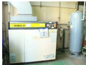
Compressor in which the pressure has been set at an appropriate level
