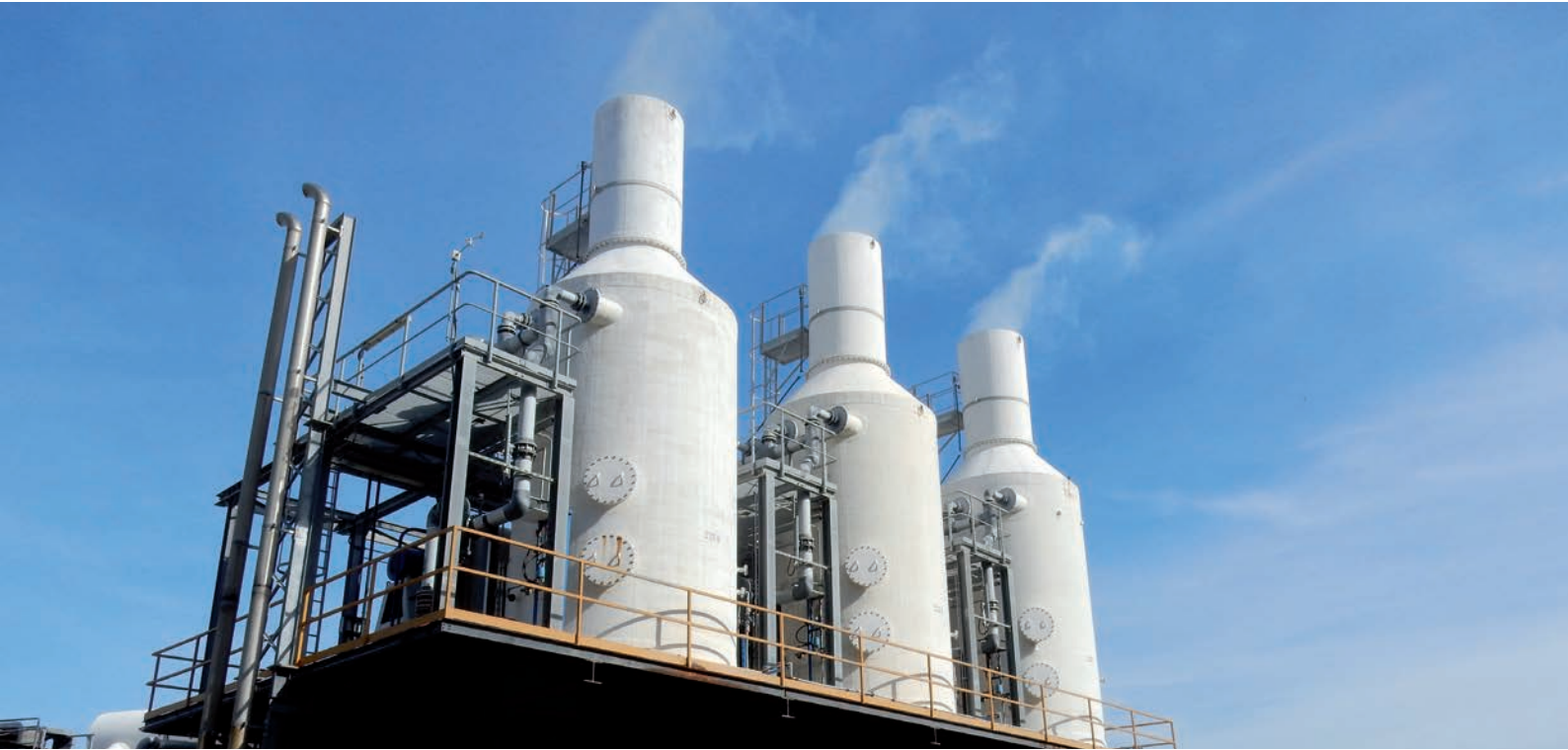
Scrubbers, ST Catania, Italy
