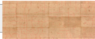
Take photographs of the concrete surfaces of bridges, piers, and tunnel for inspection. Upload the photographs to a server, and the service automatically detects highly precise images of cracks larger than 0.1 mm wide (shown as red lines). The service then automatically creates CAD data of images and crack detection results.
