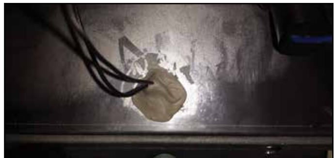
Figure 6-1.3. Sealing Compound - Door Switch (Inside)
