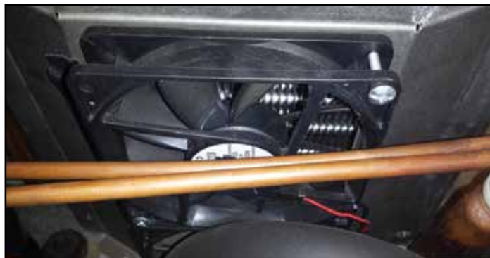
Figure 6-13. Condenser Fan Motor/Fastener
