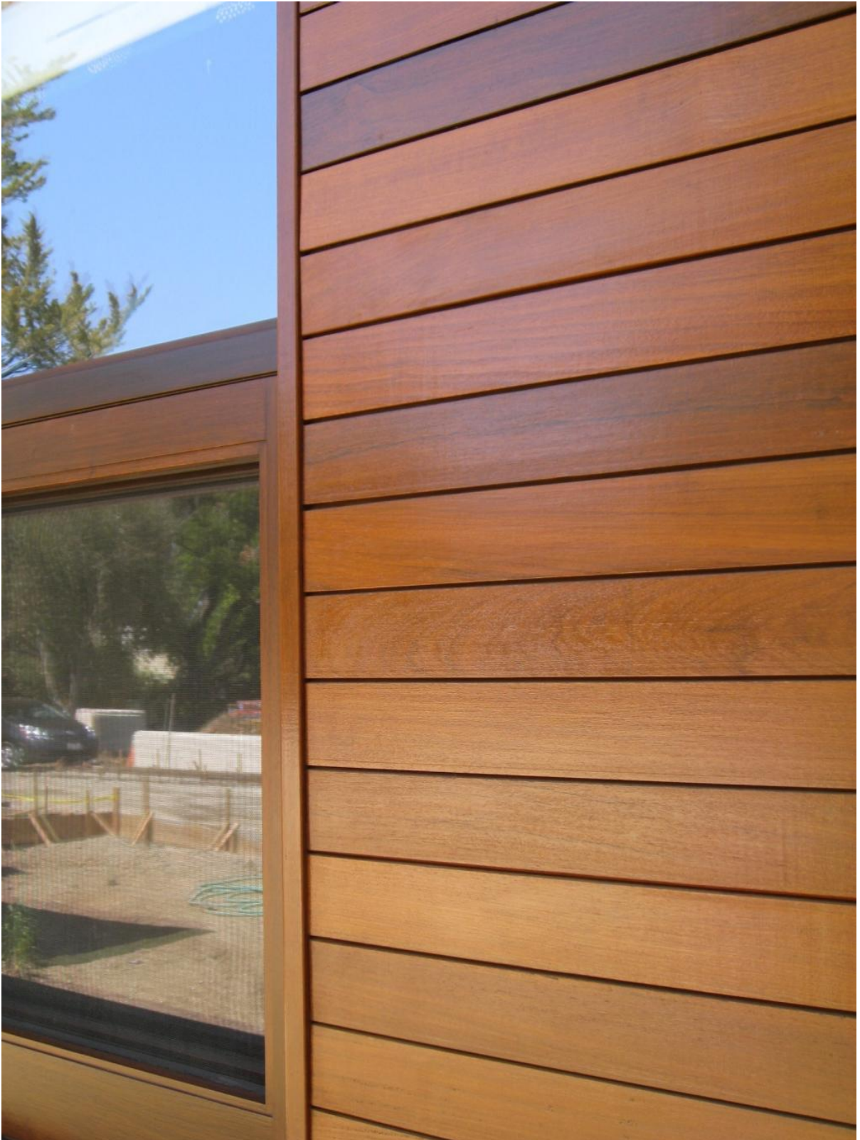
Window trim detail using 1x6 Ipe cladding in rain screen design Weeksville Heritage Center, Brooklyn New York
