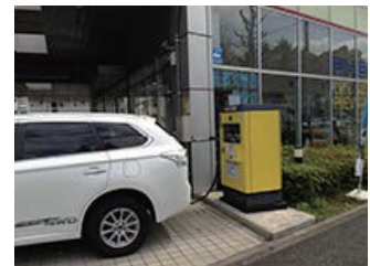
Quick charger installed in a dealer
