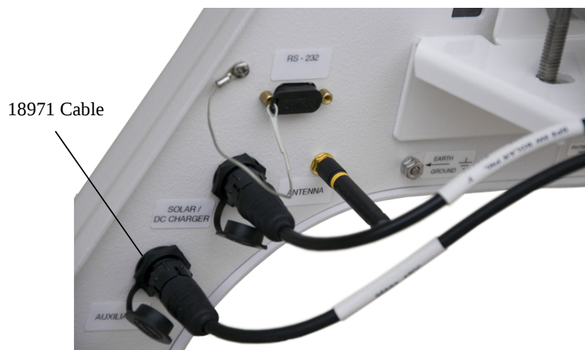
FIGURE 5-22. 18971 cable connected to TurfWeather station
