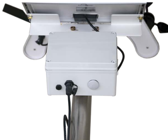
FIGURE 5-21. 18971 cable connected to auxiliary battery enclosure
