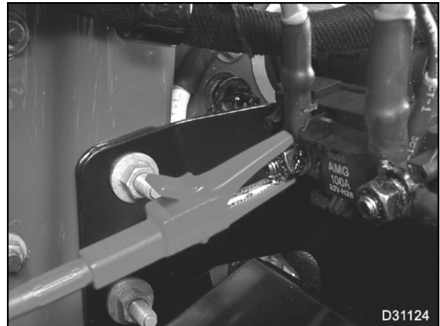
Figure 3 B+ on power distribution post
