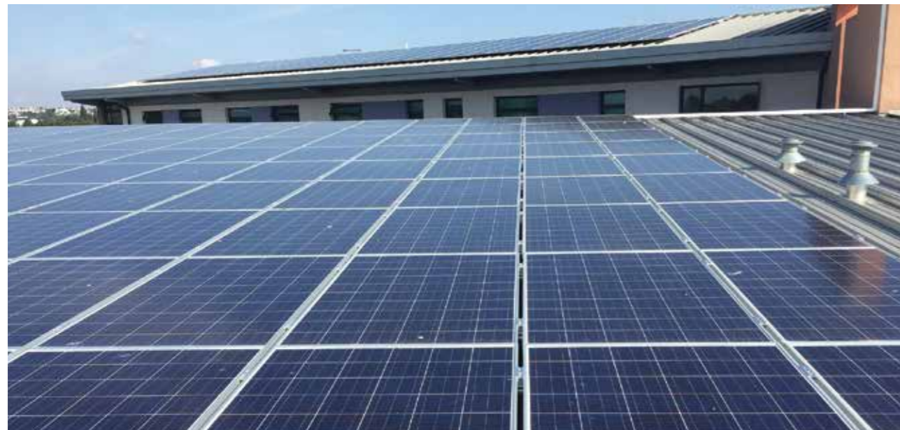
United Kingdom, 250kW United Kingdom, 250kW
