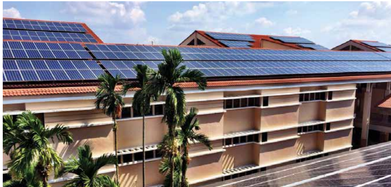
Singapore, 1MW American School
