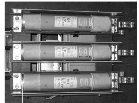
Fuse Fault Indicator
