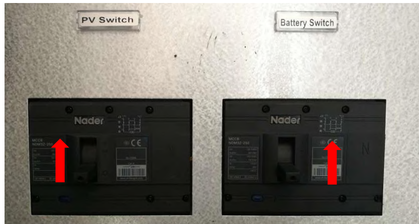
Figure 5.3 PV switch and battery switch in switch-off status
