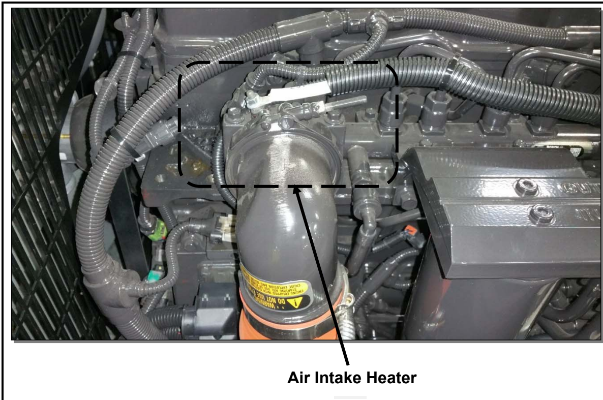
Figure 1-1-6: Air Intake Heater
